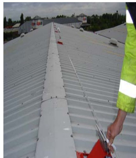
Roof Safety System
