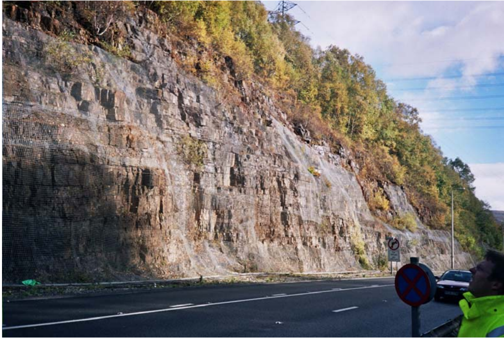
Project: A465 Heads of the Valley Road near Abergavenny Slope stabilisation measures
